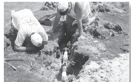
A connection to the irrigation system primes and flushes the system.
